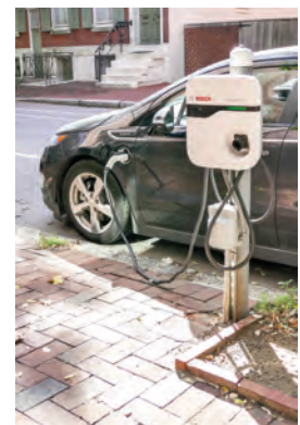
Electric car charging station
